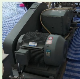
CO 2 Pump, Main pump
